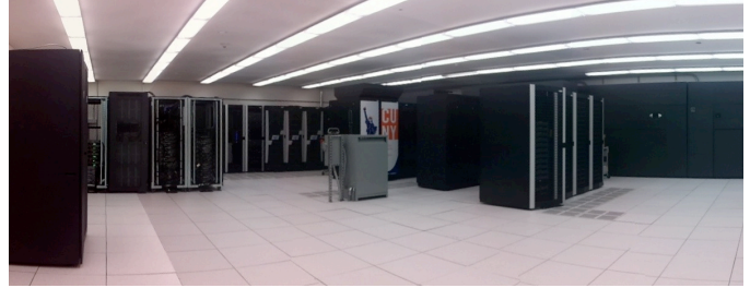
Figure 2. CUNY High Performance Computing Center facility
