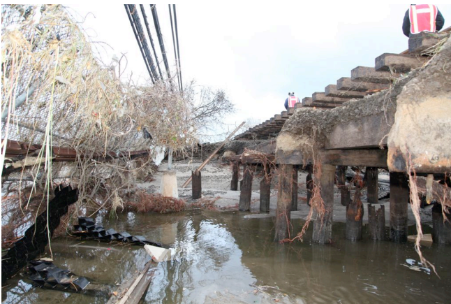
Figure 14. The subway line tracks to the Rockaways were undermined by Sandy
